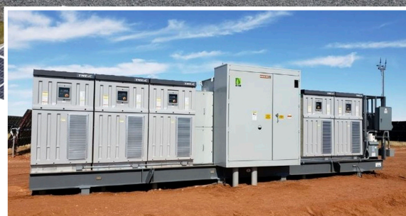
A central inverter
