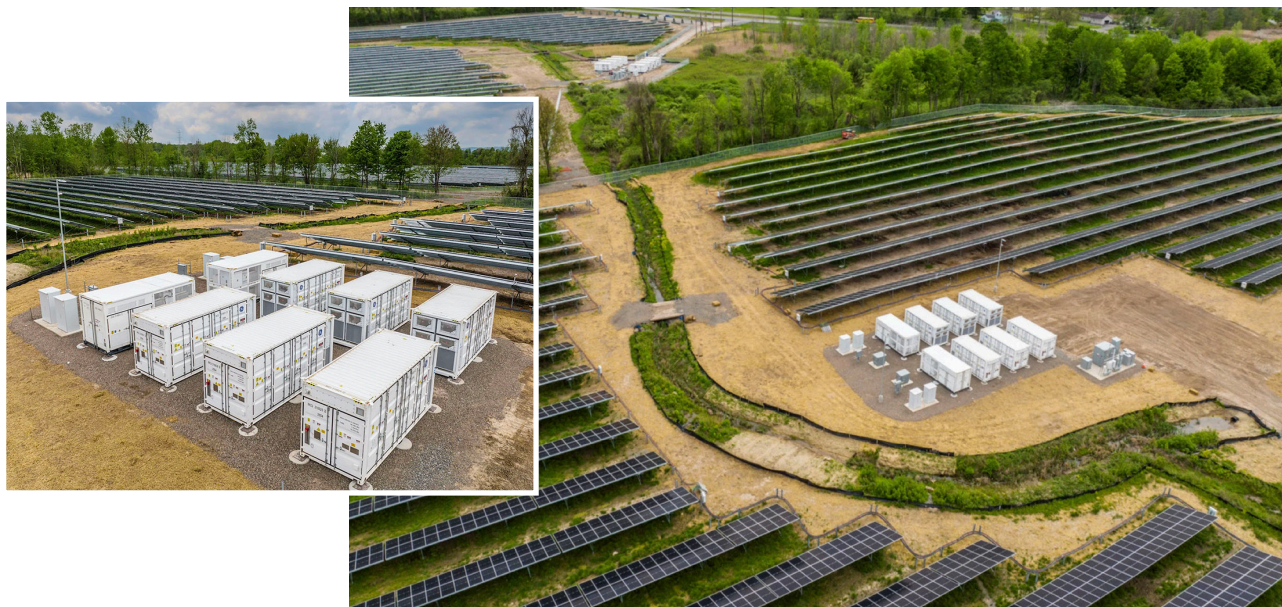
10 MW of battery storage at a 15MW solar array in Cicero, NY
