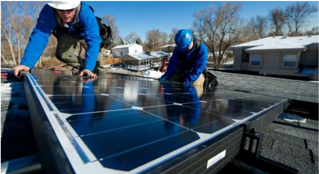
Rooftop solar installation. Photo courtesy of energy.gov
